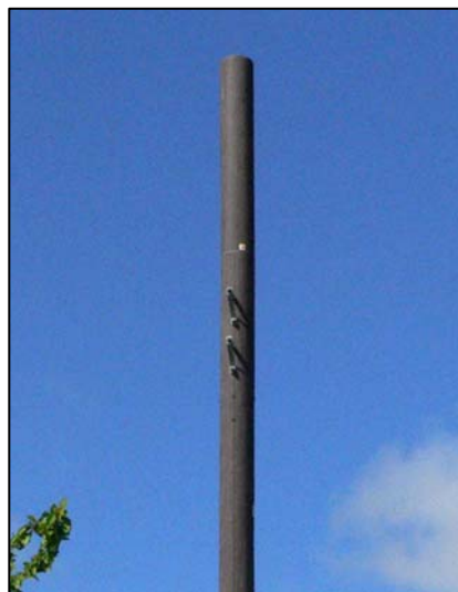
This mast on Efford Road has been designed to mimic a telegraph pole.
